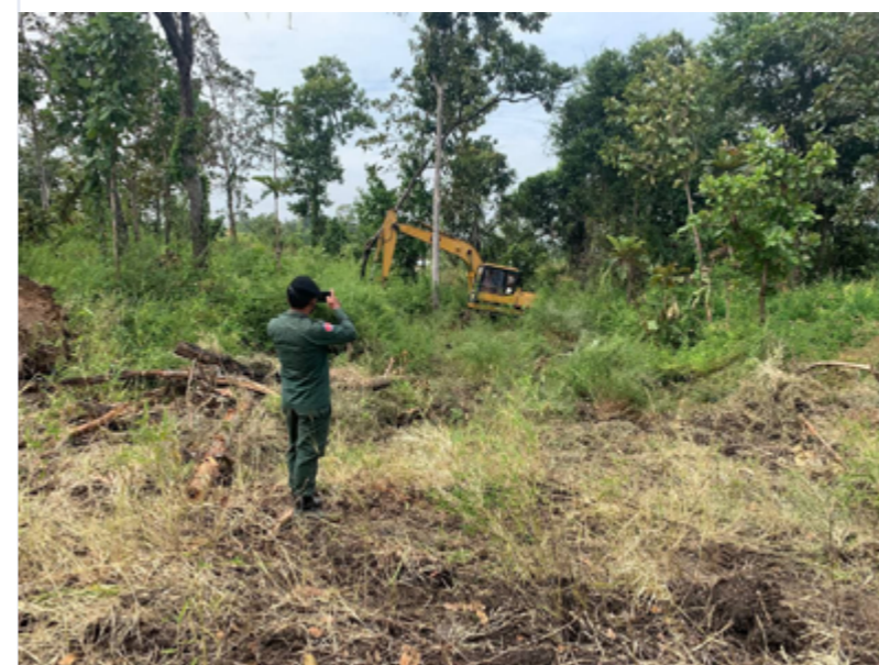
Excavators are clearing state forest land in Siem Reap Kulen district. Photo supplied
